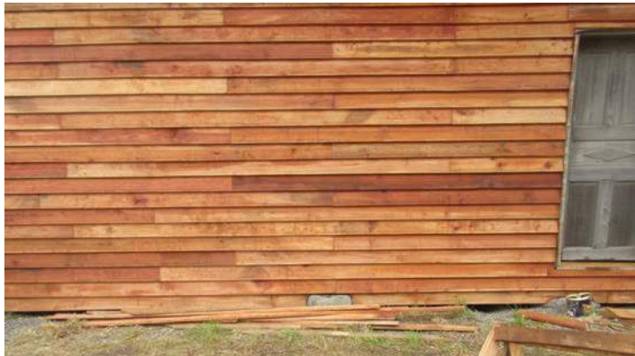
Fig. 15. Renovation of a church in San Juan with tinted Lengua as a substitute for Alerce
